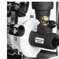
Detail of pump
